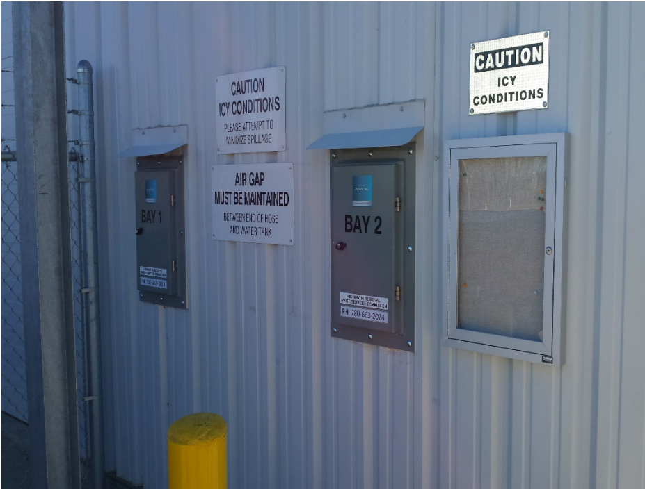
Site photograph 3: Represents the flow point access terminals.
